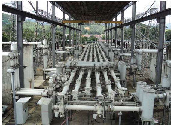
Fig. 1. Outdoor GIS at Substation Y
